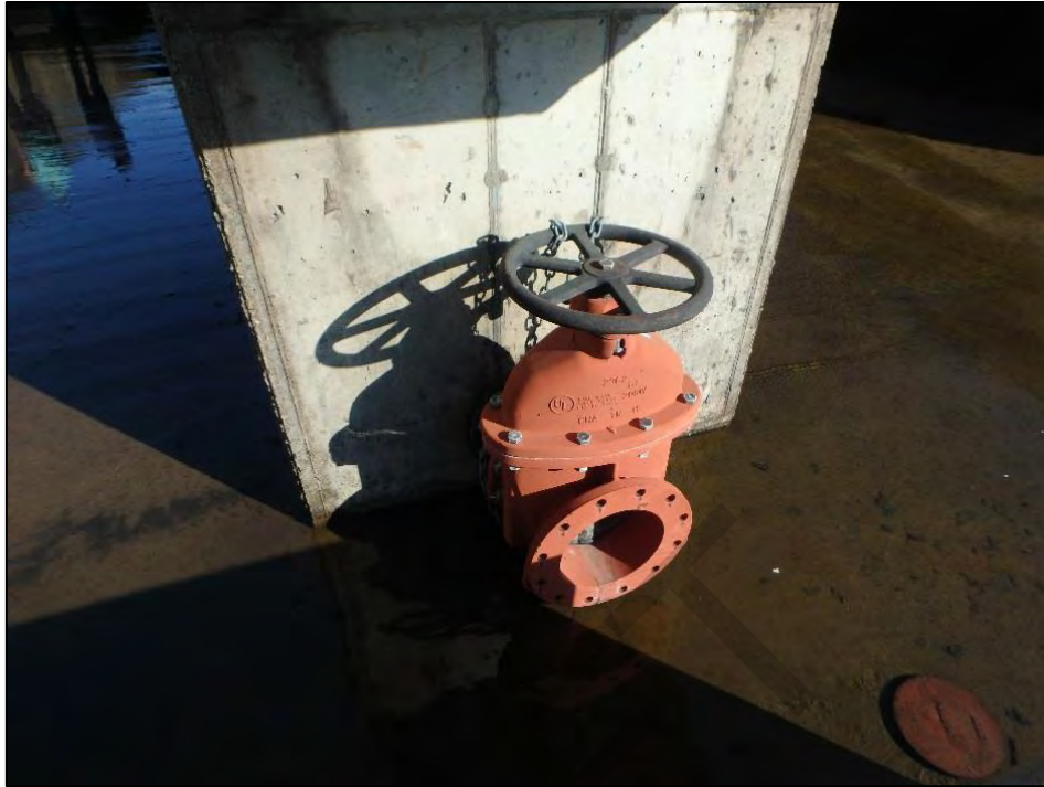
Principal spillway middle gate valve. Note operation of valve was performed at time of inspection.
